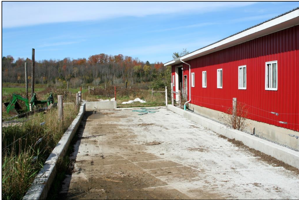
Figure 19. Two phosphorus-reduction projects completed along two Vermont tributaries of Lake Memphremagog included an improved laneway on a farm along Shalney Branch diverted barnyard and laneway runoff into the surrounding forest (upper photo) and a clean-water diversion project at a barn complex along the Wishing Well tributary (lower photo).
