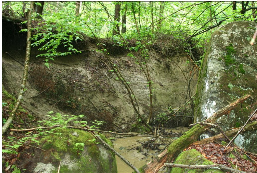
Figure 17. Extreme stream bank erosion and stream channel incision was noted along the northern branch of the Airport tributary on 9 June 2015, possibly due to excessive amounts of stormwater flowing from the Newport State Airport.
