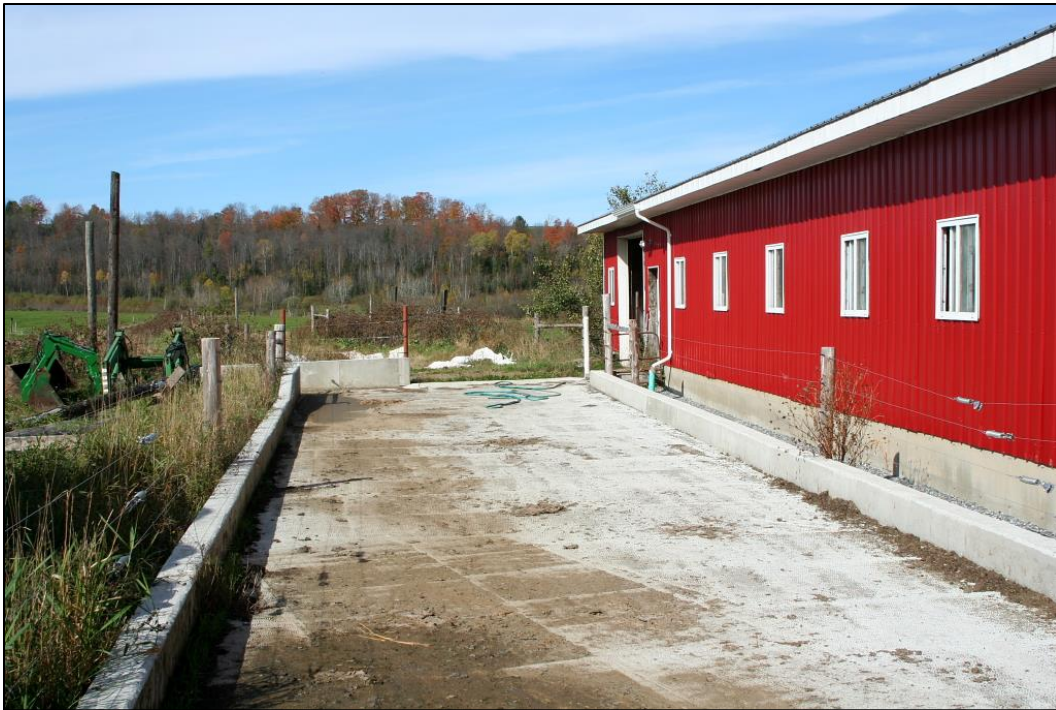
Figure 53. Clean water diversion project and concrete barnyard pad installed on a small dairy farm in the upper watershed of the Wishing Well tributary in Coventry, Vermont.
